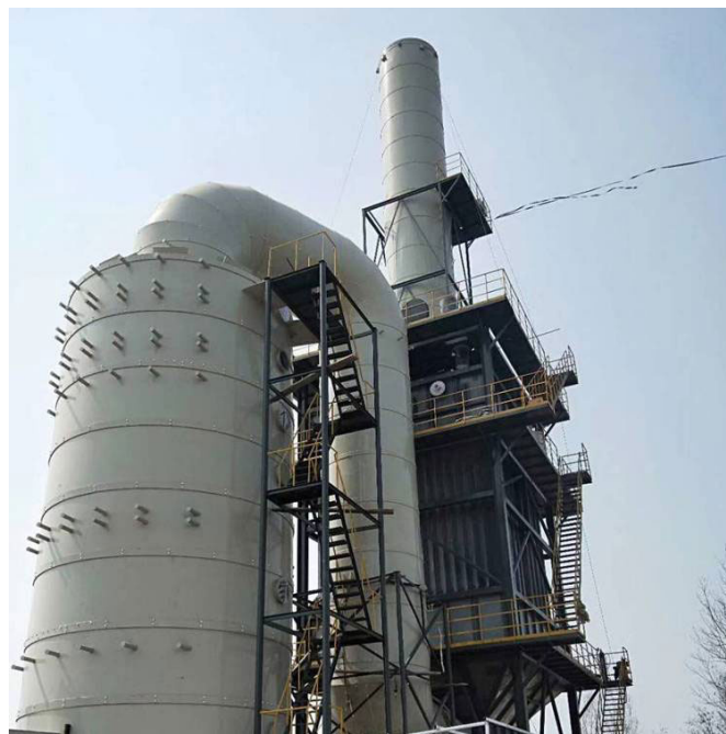
Figure A13: Sulfur removal scrubber
